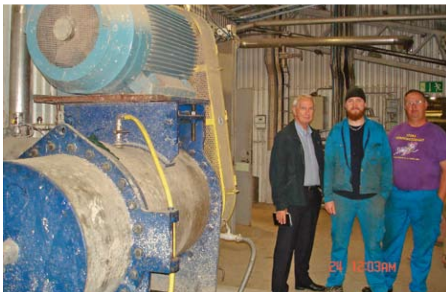
The main piece of equipment in the EcoFracSmart concept is a multifunctional pressure screen, developed by Roland Selin at JLR Pulping, seen standing to the left of 2 operators at Lagamill.
